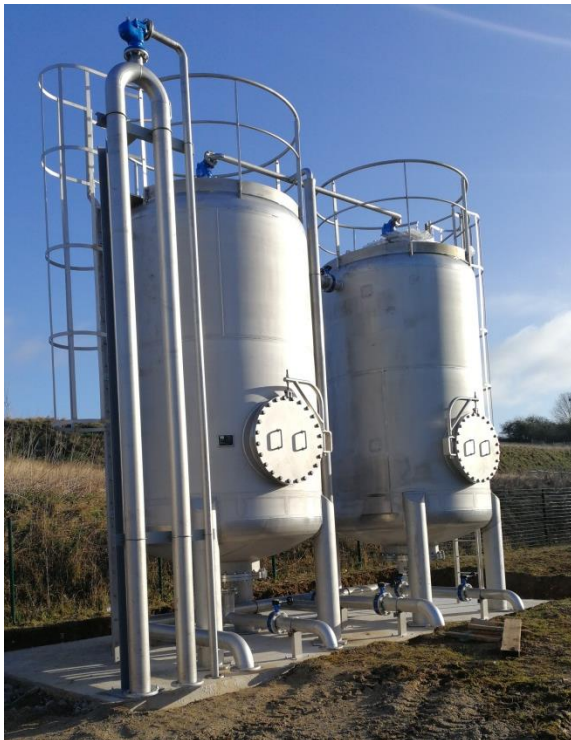
Figure 1- Tours de filtration
